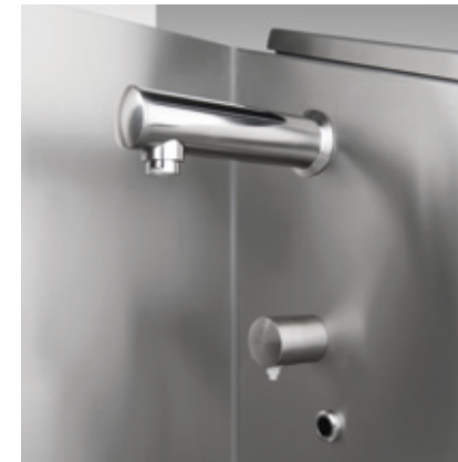
Detail: Outlet tap and soap dispenser
