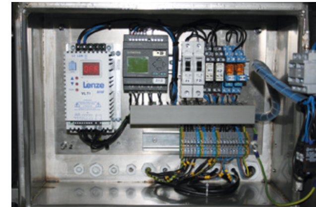
High-quality control cabinet components
