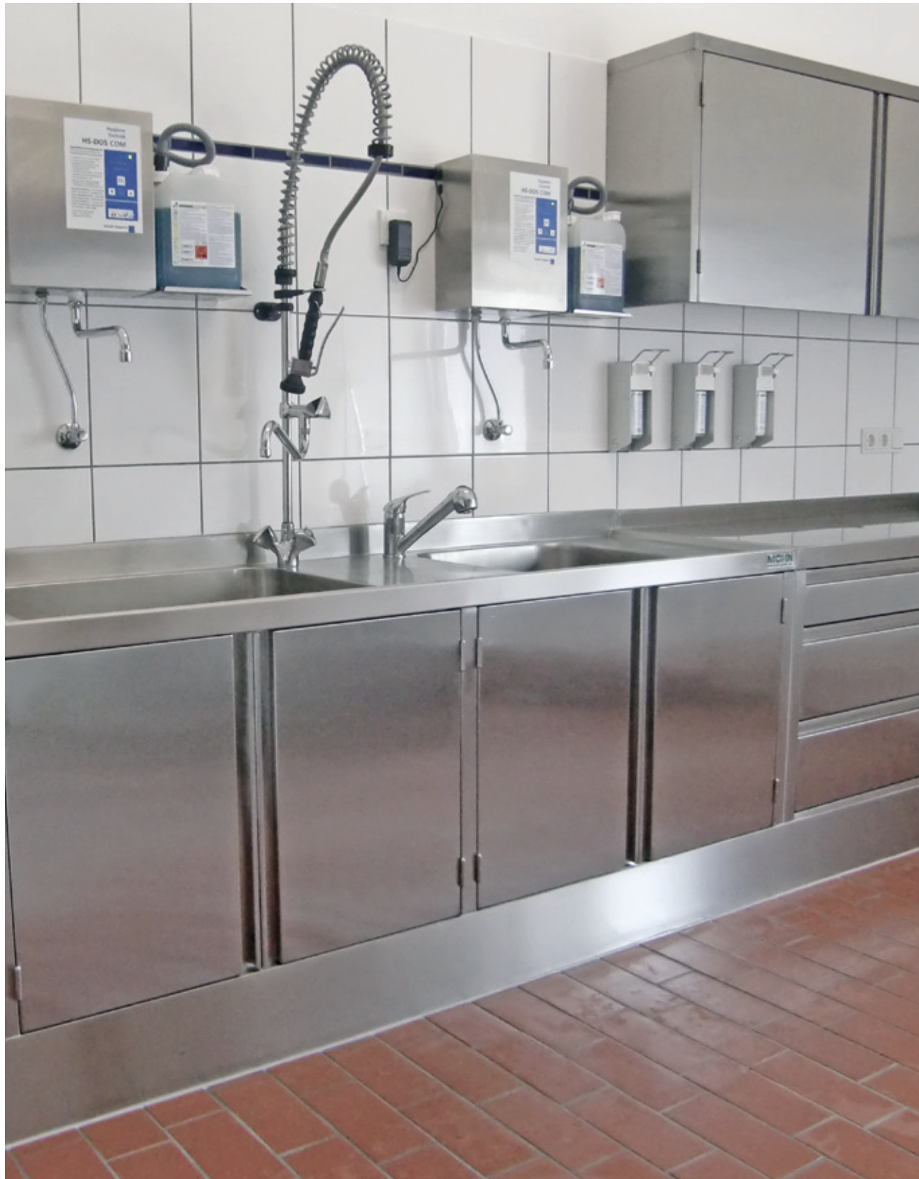
Kitchen units and work cupboards with wall-mounted cupboard
